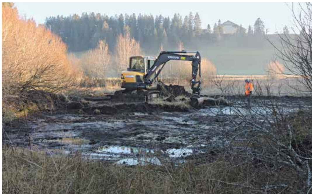
Machines at work for nature: a digger is building dams and excavating ponds to re-wet the bog (photo: Yvan Matthey).
