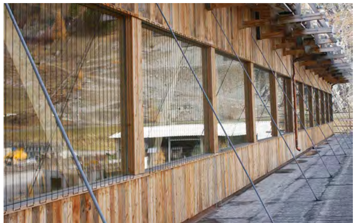
After repeated bird collisions with the reflective windows of a factory building in S-chanf, Switzerland, black nylon cords were put up at 8-10 cm intervals. No further bird collisions were recorded after the retrofitting.
