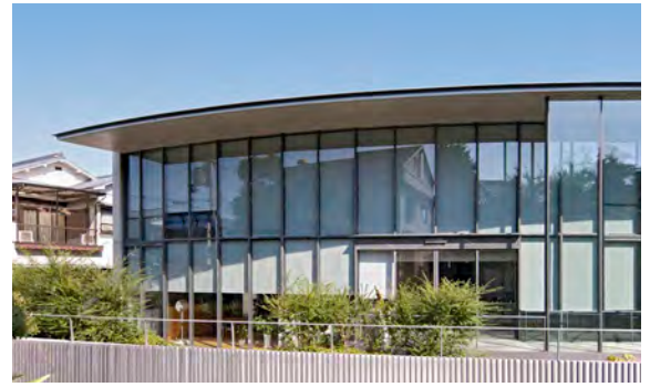
Although interior blinds and light-coloured curtains behind the windows can reduce reflections, they often still occur. Such measures cannot be expected to provide effective protection against collisions, especially as blinds are not permanently closed.
