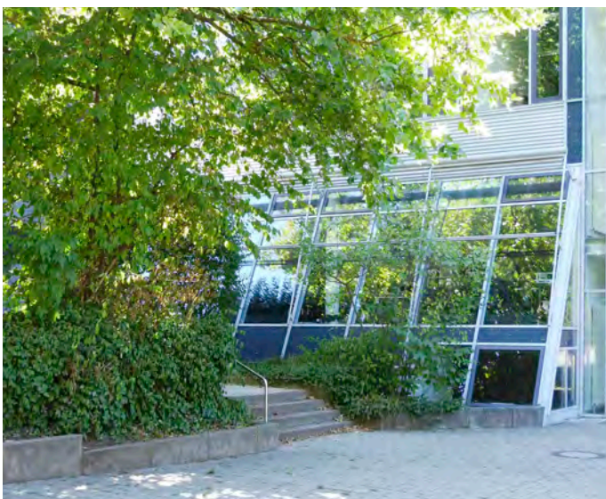
The reflections on this sloping glass façade of a school building are just as clear as on a vertical pane and thus pose a high risk of collision.
